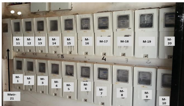
Fig. 5. Typical cluster of electricity meters in a 4-levels (21 meters).
